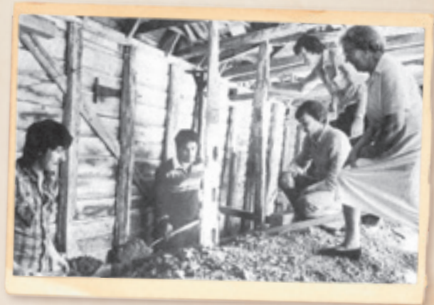
The restoration of a 120-year-old milking shed in Wilton, Wellington, is an example of the interesting work being carried out by members of the Work Skills Development Programme. Photo: Evening Post. Appeared in War Cry, 15 May, 1982.
